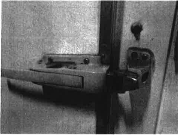
Seal/Handle Adjusted on Manual Door to Freezer
